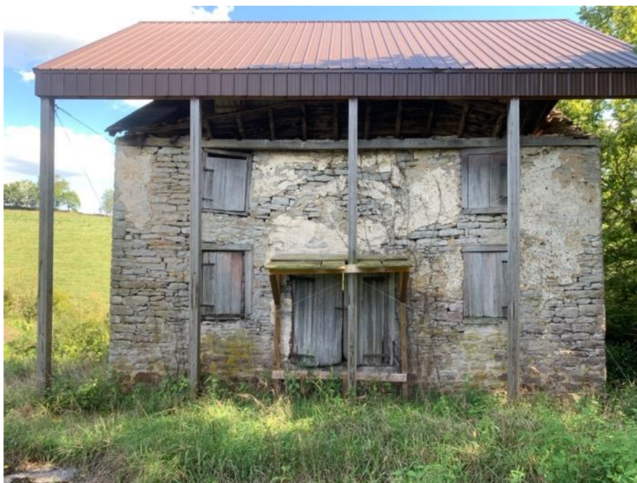
Figure 43. The north-facing wall of the surviving dormitory of the Choctaw Academy, built c. 1825. Photo by the author.
